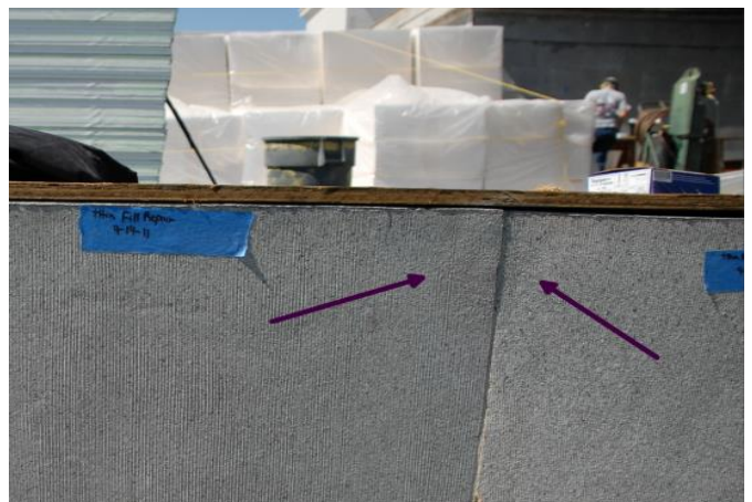
Before and After: Glazed terra cotta spall (top), filled and smoothed using THIN-FILL 55 prior to glazing and speckling with AQUATHANE UA210 and AQUASPEX 220 coatings (bottom), matched to original glaze colors. Project is California State Library in Sacramento, CA.
