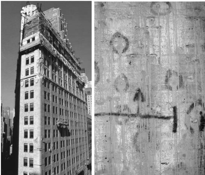
Figure 3 (left): Pump-X53 was used to fill voids between terra cotta band courses and rubble masonry backup on this project in New York City. Figure 4 (right): Injection points are marked on an interior wall surface; Pump-X53i was injected through the back-up wall into the masonry exterior veneer to fill cracks and voids in the stonework.
