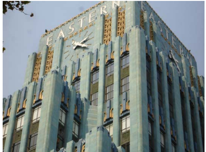
Figure 6: Multiple colors of Aquathane UA210E coatings were custom-matched to the polychrome terra cotta at this landmark building in California.
