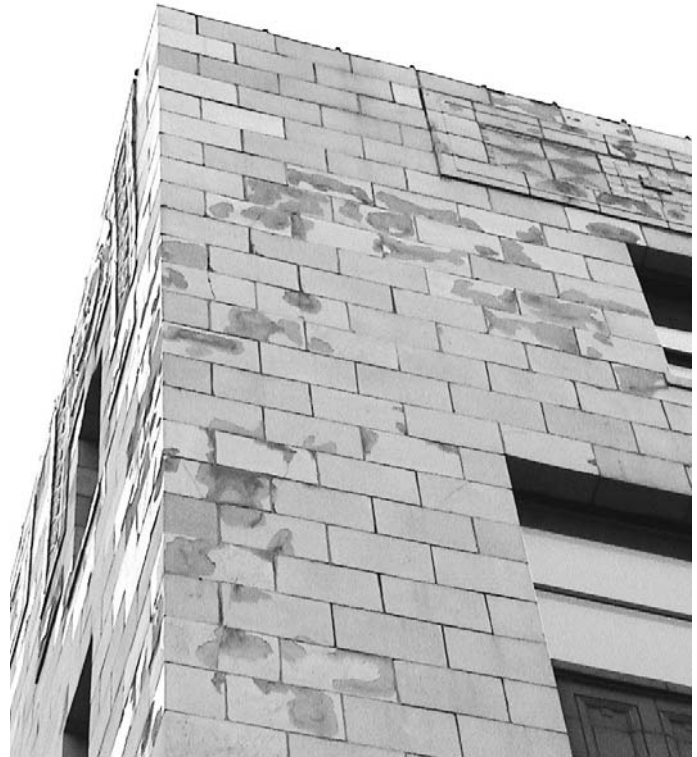
Figure 2: Thin-Section glaze spalls are common in terra cotta subjected to bulk moisture infiltration.
