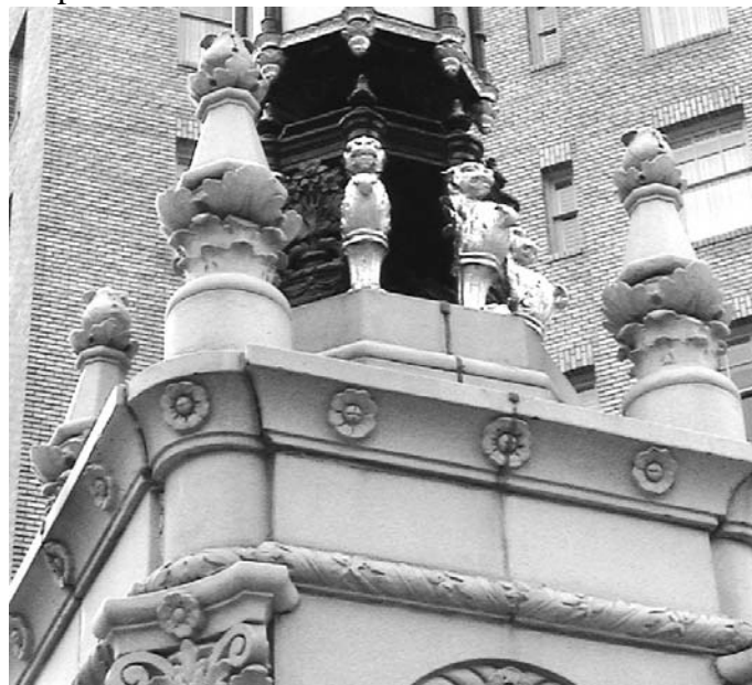
Figure 1: Replacement finial (right) was cast with custom color-matched Custom System 45 using Restoration Latex RL-2.
