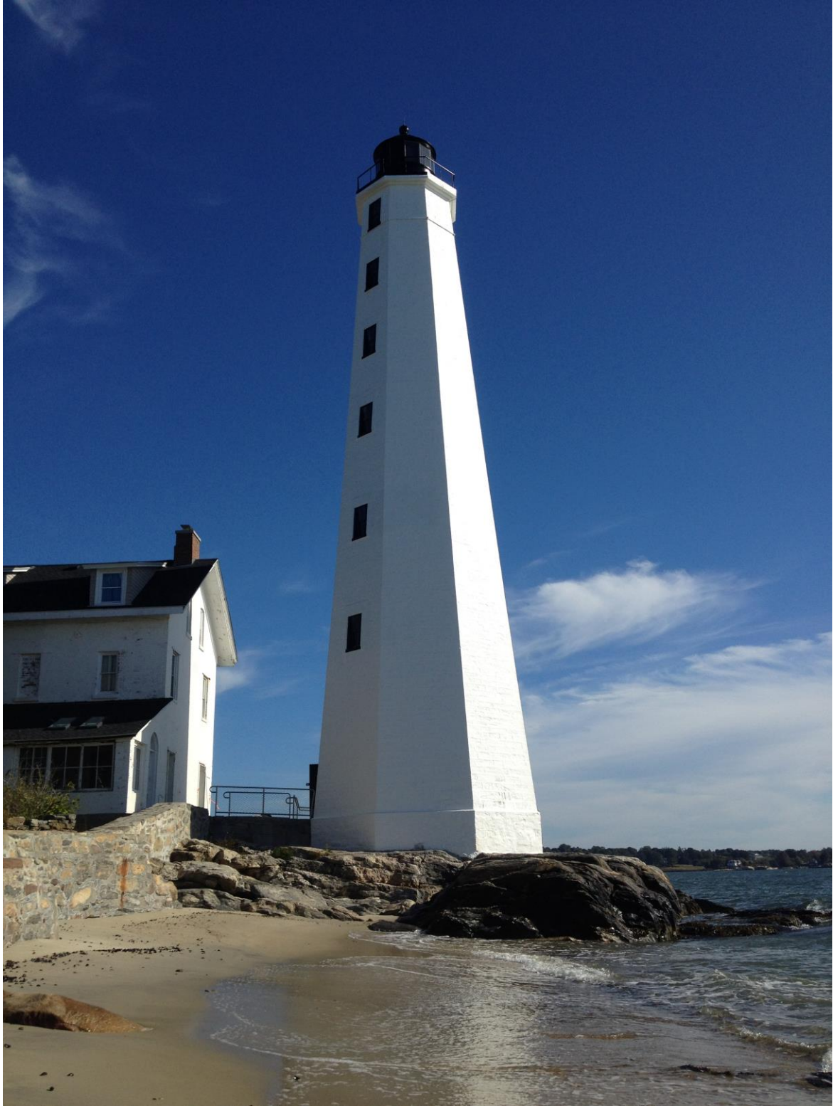
Masonry restoration and coating work was performed by Loring and Son Masonry of New London. All photos courtesy of Loring & Son Masonry, Inc.
