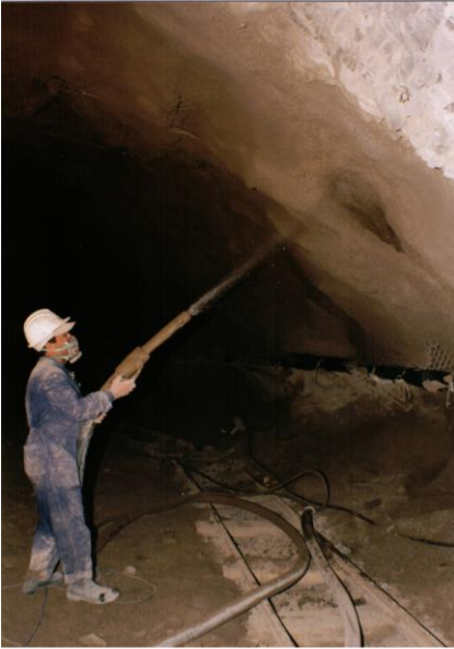
MARFIL may be used in a wide variety of applications using an array of different equipment and methods. PHOTO: Shotcreting in a subterranean tunnel.
