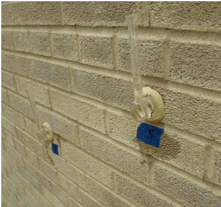
3. RILEM tube testing can be performed to assess mortar's water absorption rate. Excessive absorption can be an indication of improper placement, compaction and/or curing.
